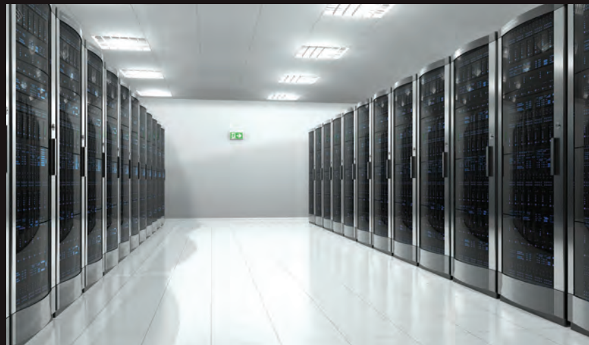
DRT 8MW Data Centre London
