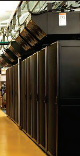
0MW Data Centre, Dublin
