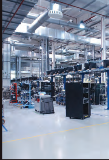
IBM 1.5MW Data Centre Dublin
