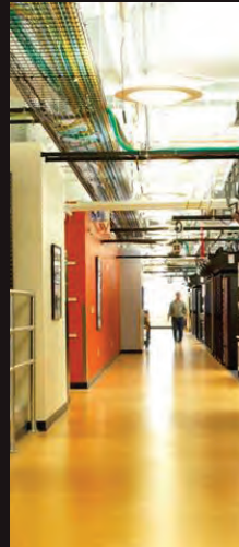
Data Electronics 10MW
