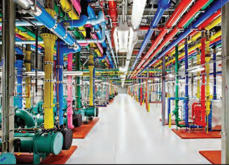
32MW Data Centre Finland
